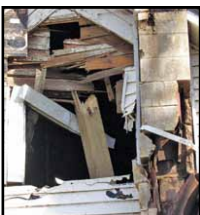
Many homes in rural areas in Wayne County were destroyed or damaged, including here at the Larry Haase residence.
